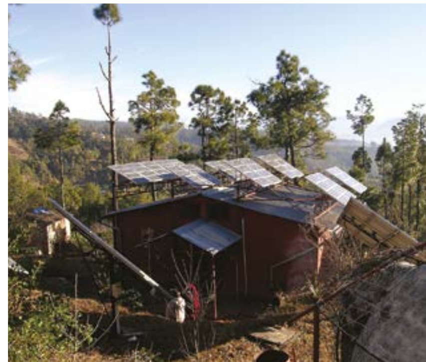
Above and Left: Solar electrified village and AVANI solar power plant.
